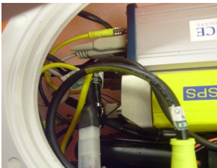
(Fig. 4.28) Position all access wiring in the space behind the instruments
